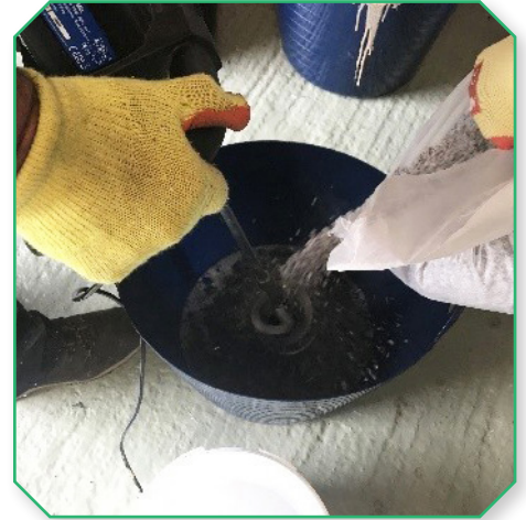
Use large bucket for mixing. Power drill with paddle to be used for mixing.
